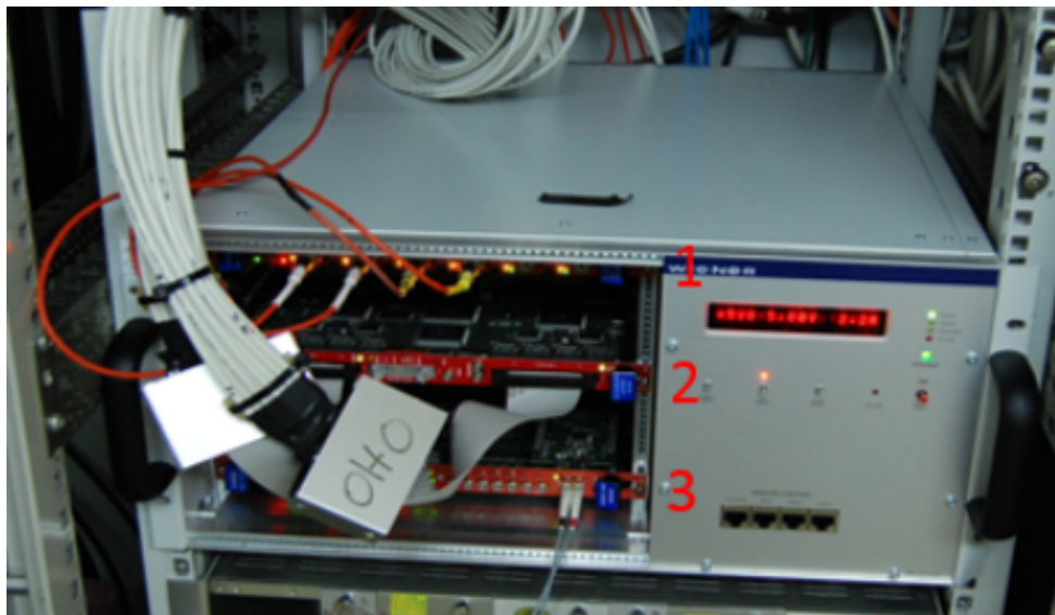
Figure 3.9: In this photograph we can see the card with high voltage for the PMT (1), the cables from the OB with digital signal connected to the CAEN counter card(2) and the communication cable of optical fiber from CAEN to labm-computer (3).
